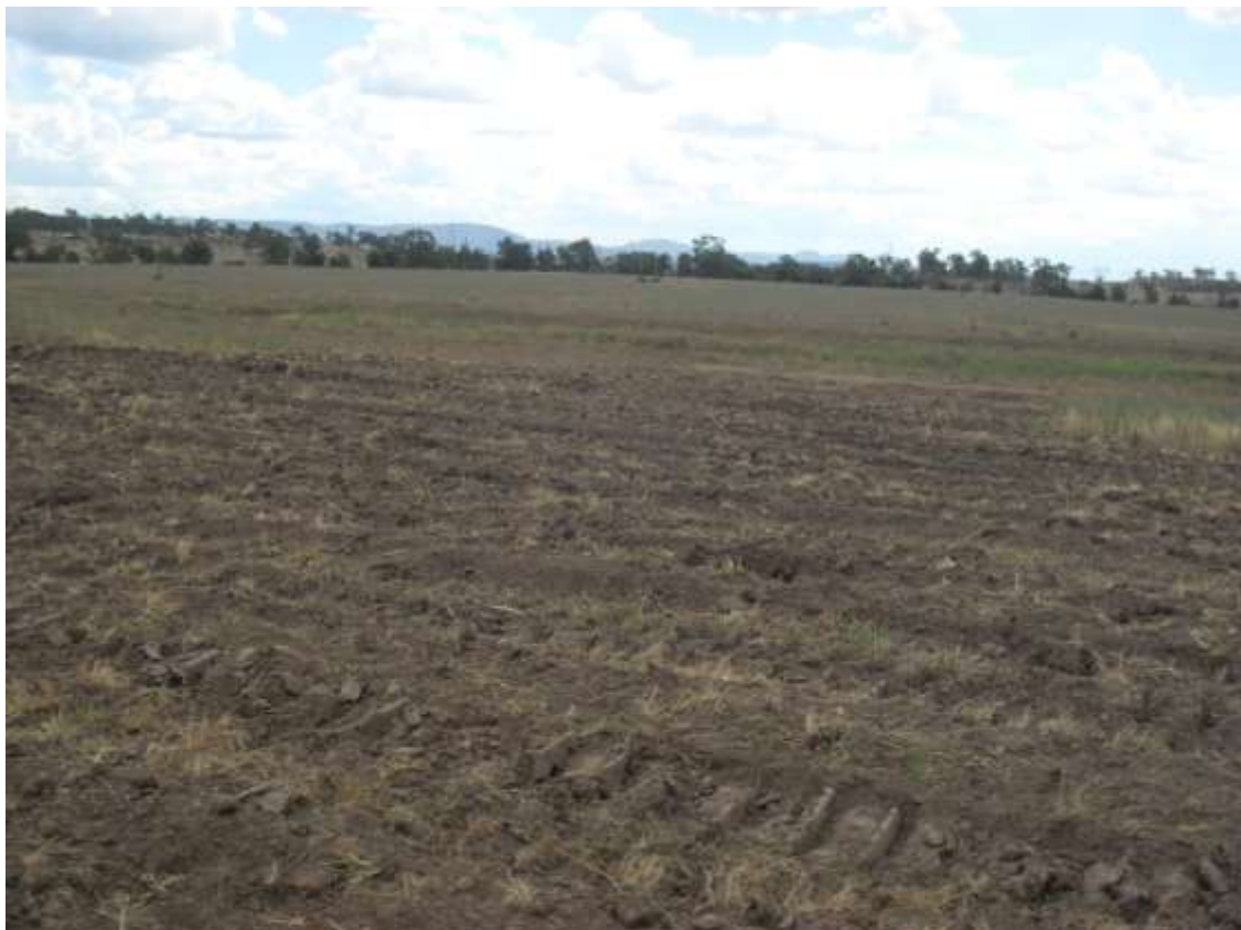
Figure 7: LW6A start line remediation post remediation on 02/02/2011. This photo looks from the tailgate corner to towards the centreline (south-west).
