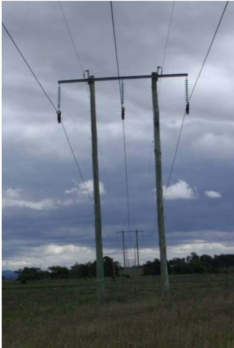
Figure 4: 2-pole 132kV power line located mid panel in LW6A (Chainage 985m) looking west from 05/04/2011.
