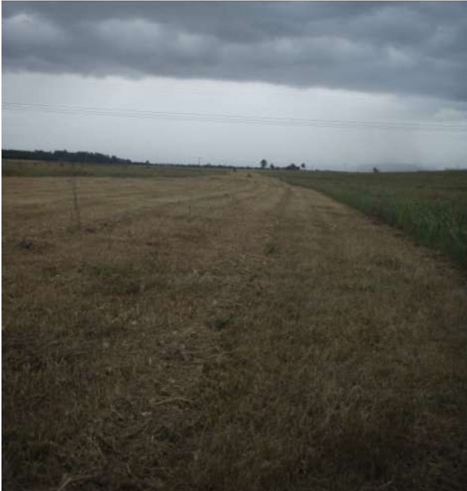
Figure 5: Location of gateroad cracking looking north. Gateroad cracking over the Maingate was concealed by heavy grass growth. Slashing occurred prior to remediation to help locate all gateroad cracks in the area.
