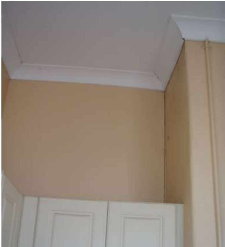
Figure 8: Cracking between the wall and cornice in the 'yellow house'. The shown cracking is the worst observed from within the dwelling post subsidence.
