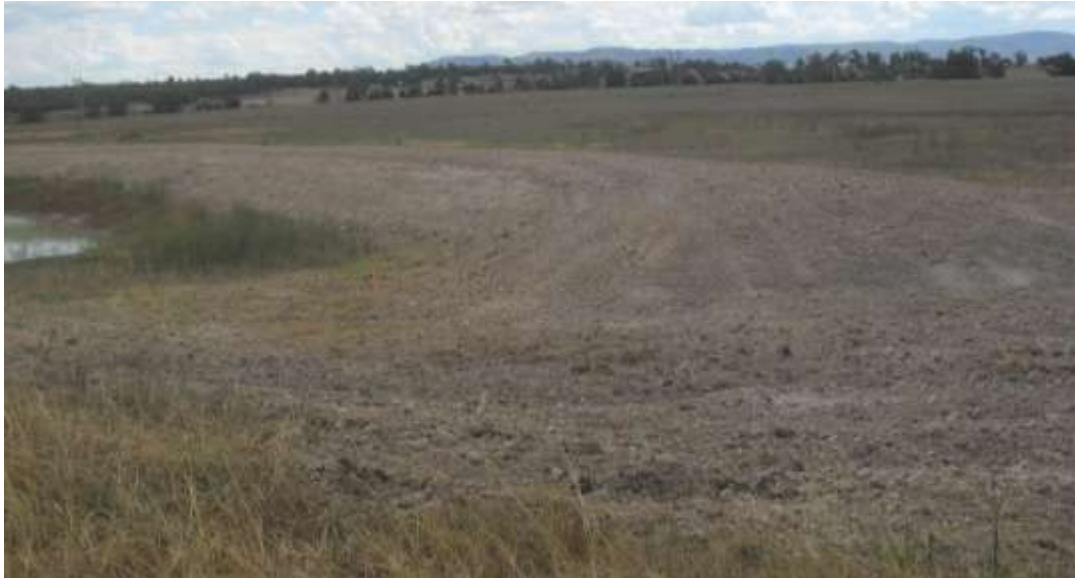
Figure 10: Dam 10 post wall re-profiling. The dam wall was re-profiled so that the lowest point of the dam was again the spillway as designed. This was taken on the 02/02/2011 and is looking south-south west (Ref: Figure 9 ).
